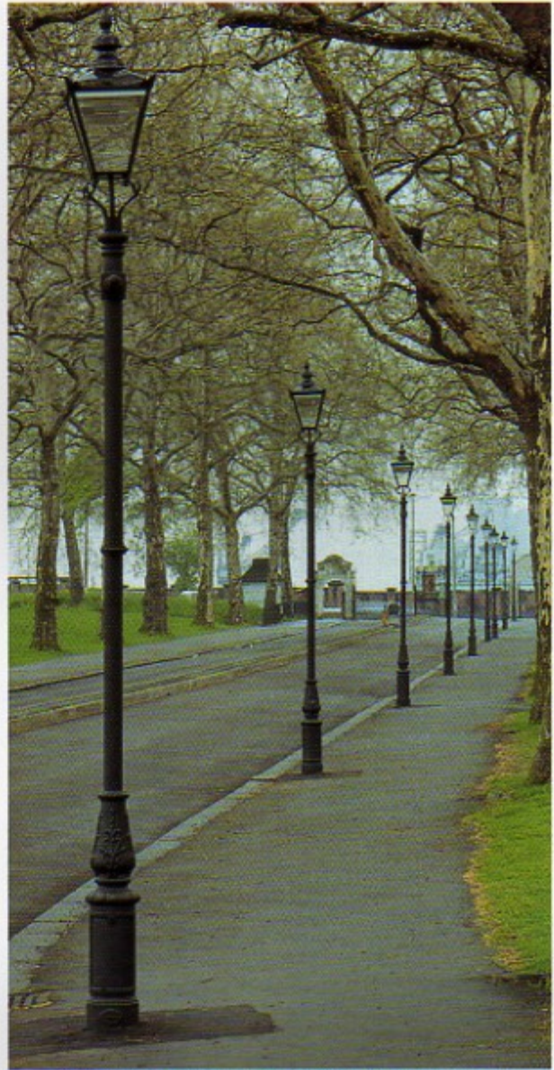
DW Windsor lanterns on Oxford lamp posts line a road through a park.
