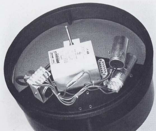
Canopy removed for access to gear department
